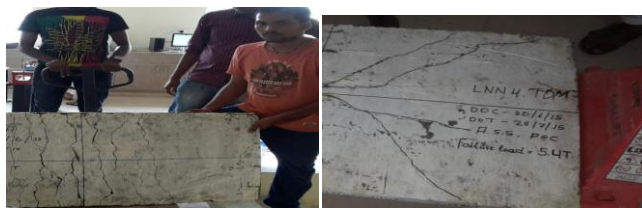
Crack pattern for S5 and S6 slabs
